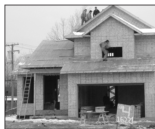
By providing hands on experience for students, the building trade builds an entire house every year.
